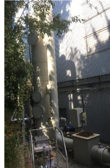
Water scrubber and heater
